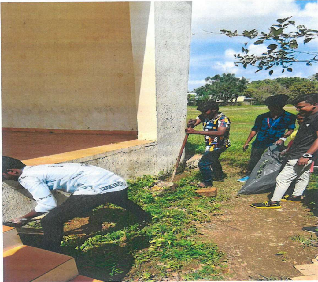
Students are repairing the halt places in the village camp, Salavakkam from 23/12/2019 to 29/12/2019
